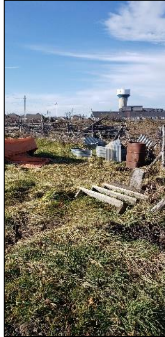
Image 5. View of the construction material located within the construction yard, facing northwest. (20201109_134932)
