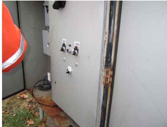
Photo 27: Robert Street SPS – Electrical panel installed in the 1970s
