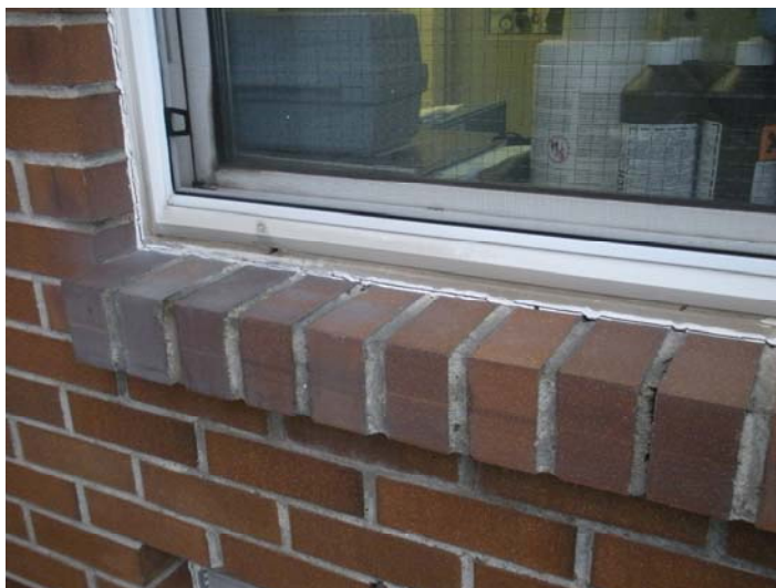
Photo 16: Wells 7 and 8 - Cracked caulking
