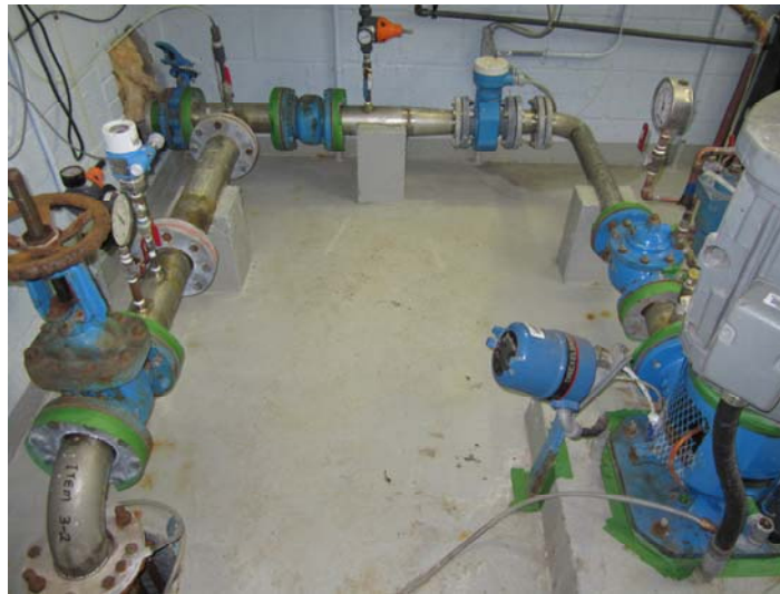
Photo 4: Well 3 - Unprotected carbon steel bolts
