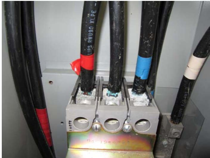
Photo 14: Well 6 - Severe corrosion on the line side wiring of the main disconnect box
