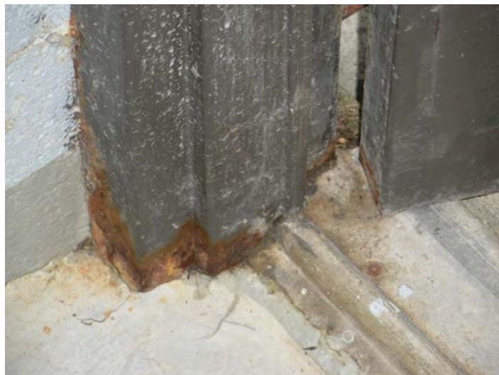
Photo 2: Well 3 - Corrosion on door frame base
