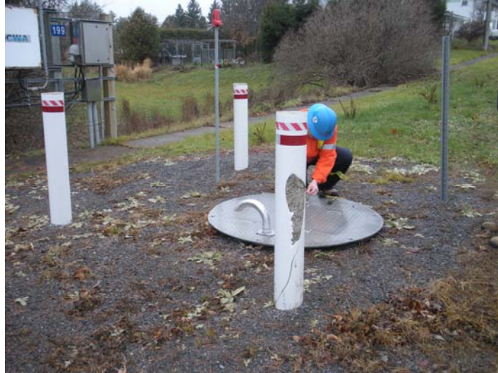
Photo 20: Christian Street SPS - Damaged bollard
