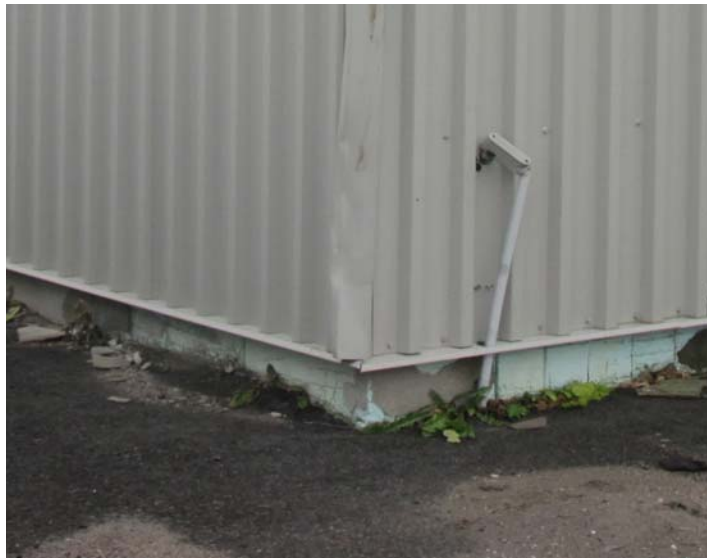
Photo 11: Well 5 - Damaged conduit
