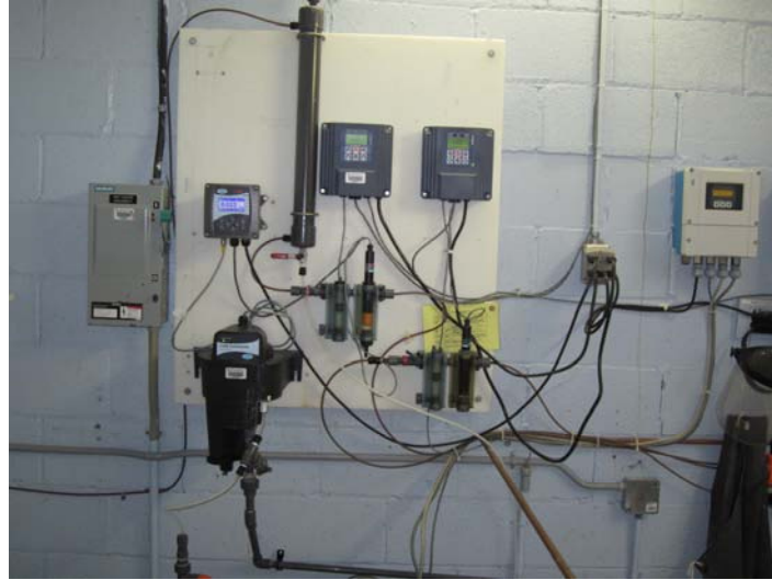
Photo 5: Well 3 - Flexible tubing appears to have too much slack
