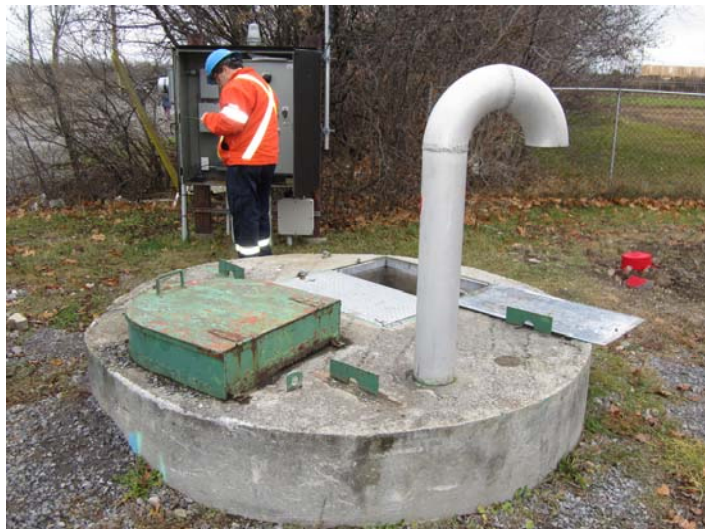
Photo 25: Robert Street SPS - Corroded access hatch cover
