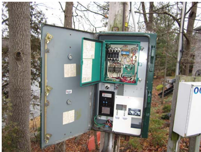
Photo 23: Hope and Glass Streets SPS - Electrical panels installed in the 1970s
