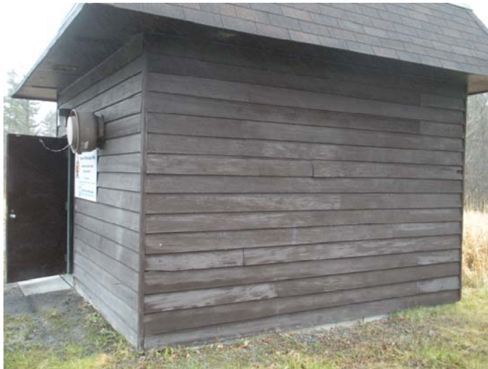
Photo 12: Well 6 - Exterior siding has reached the end of its useful life
