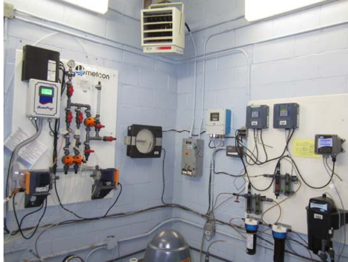
Photo 9: Well 5 - Tubing in the chemical injection / water sampling systems with slack
