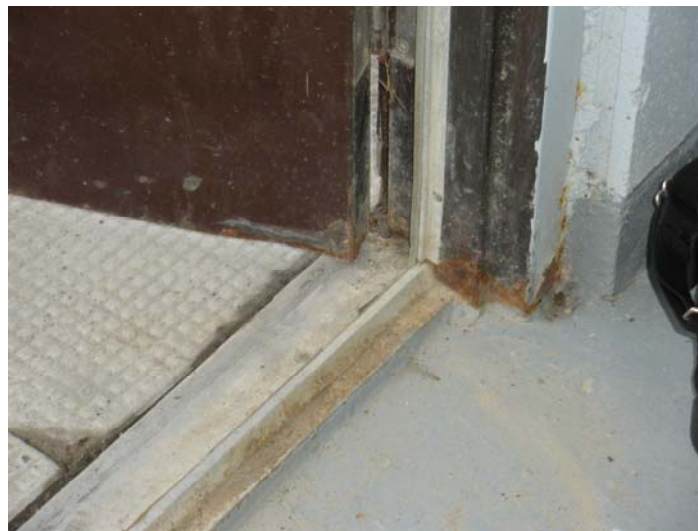
Photo 13: Well 6 - Corrosion at base of door and frame
