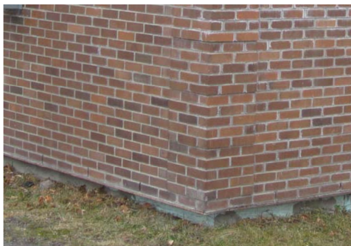
Photo 3: Well 3 - Cracked parging
