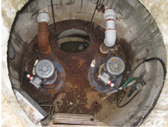
Photo 22: Hope and Glass Streets SPS - Surface rust on the steel discharge pipes
