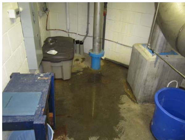
Photo 18: Elevated Storage Tank – Electrical clearance and water ponding concern
