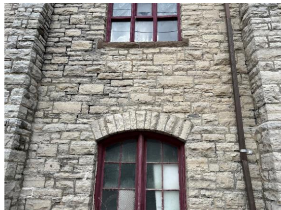
Photo 18: Localized Voids in Mortar joints in South Wall
