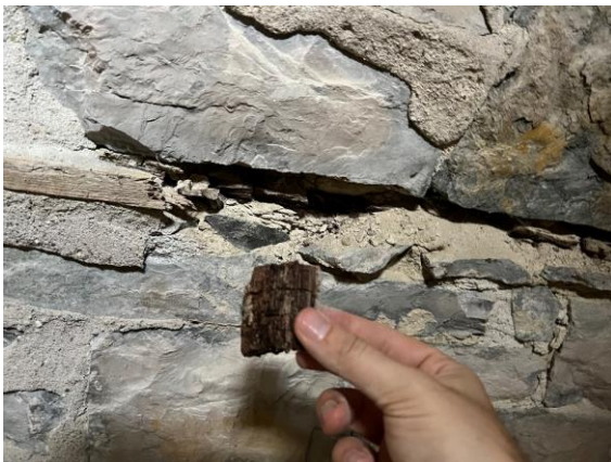
Photo 7: Rotting Wood Nailer in Belltower
