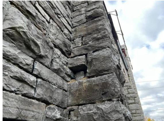
Photo 20: Missing Stone Unit in Buttress
