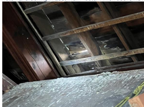
Photo 14: Water Staining and Natural Light
