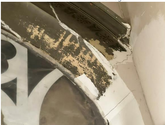
Photo 13: Cracking in Plaster Finish at Window
