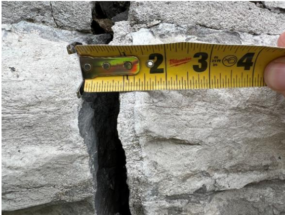
Photo 5: Large Vertical Cracking
