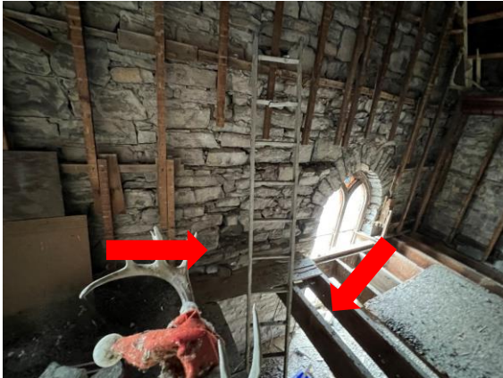
Photo 15: West Wall in Poor Condition with Voids and Stone on Ceiling Below
