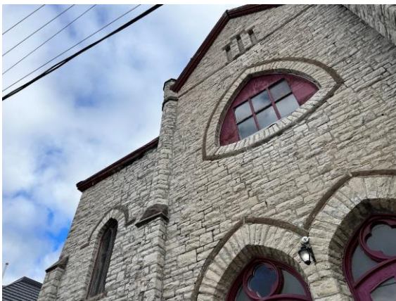
Photo 17: Localized Voids in Mortar joints in West Wall
