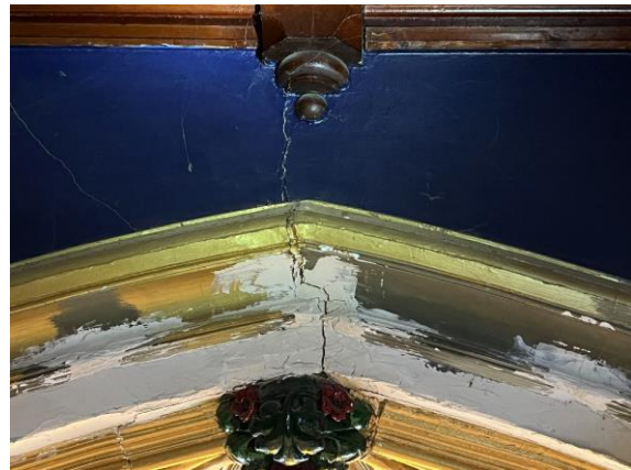
Photo 12: Cracking in East Wall Plaster Finish above Nave
