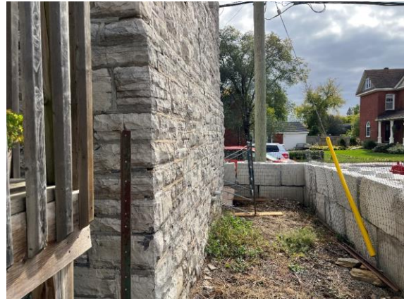
Photo 6: Significant Bow in Exterior Wythe
