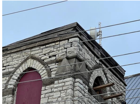
Photo 10: Southeast Corner in Poor Condition
