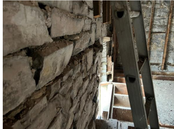
Photo 16: Displaced Stone in West Wall
