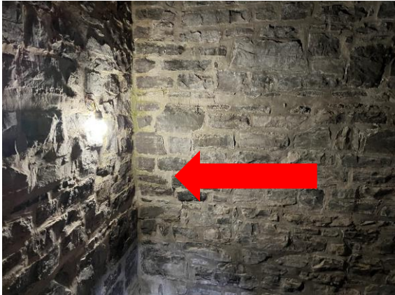
Photo 2: Cracking in Interior Wythe
