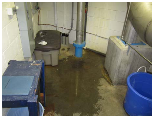
Photo 18: Elevated Storage Tank – Electrical clearance and water ponding concern
