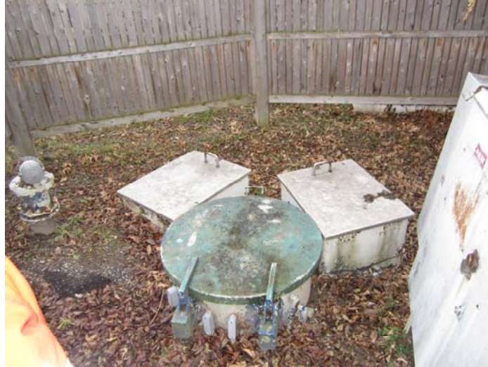
Photo 24: Island SPS - Corrosion on exposed access hatches
