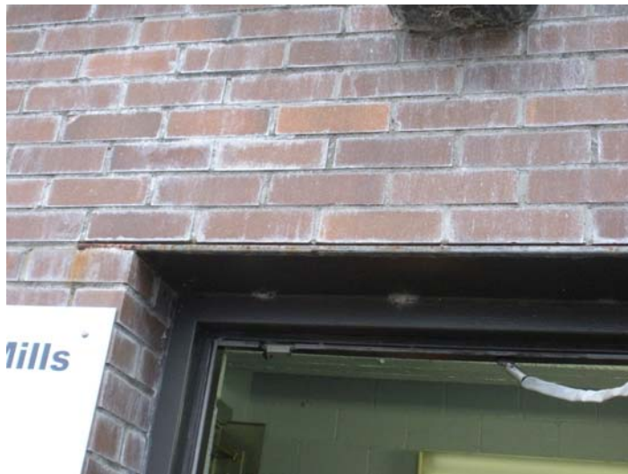
Photo 1: Well 3 - Efflorescence on exterior brick
