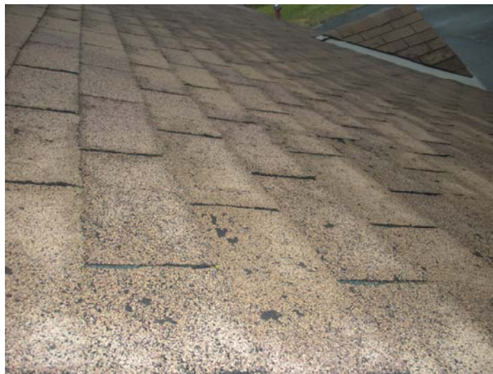
Photo 15: Wells 7 and 8 - Asphalt roof shingles starting to fail
