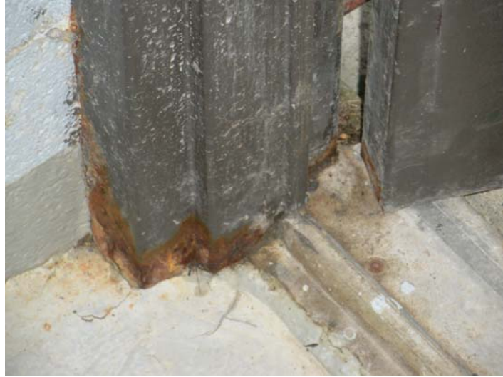
Photo 2: Well 3 - Corrosion on door frame base
