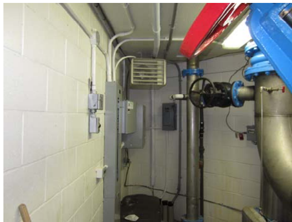
Photo 17: Elevated Storage Tank – Electrical clearance and water ponding concern
