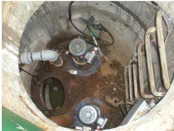
Photo 21: Hope and Glass Streets SPS - Surface corrosion on checkerplate
