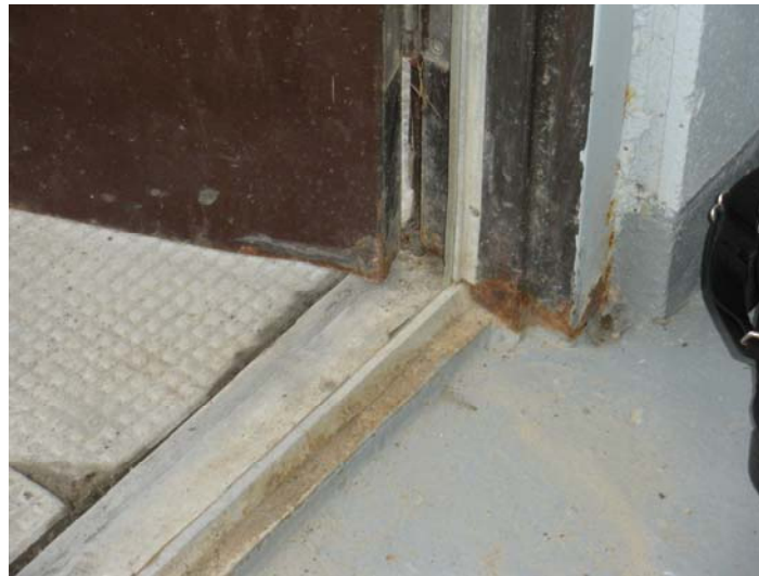
Photo 13: Well 6 - Corrosion at base of door and frame
