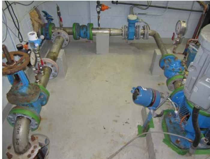
Photo 4: Well 3 - Unprotected carbon steel bolts
