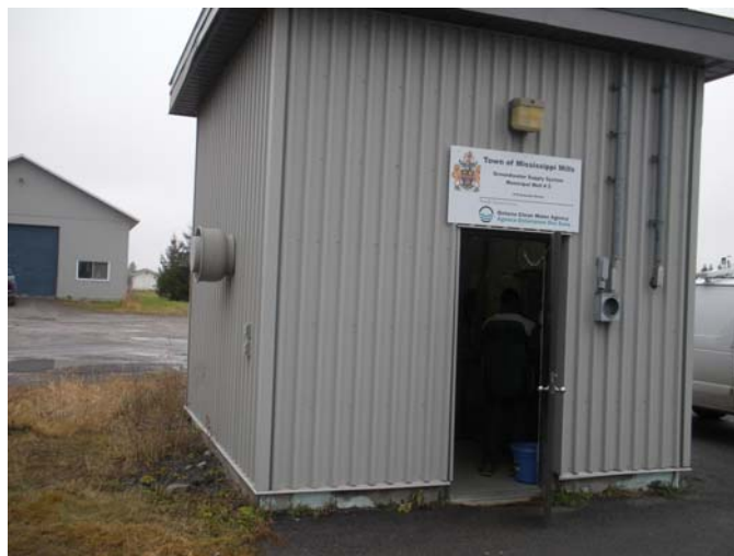
Photo 7: Well 5 - Poor drainage
