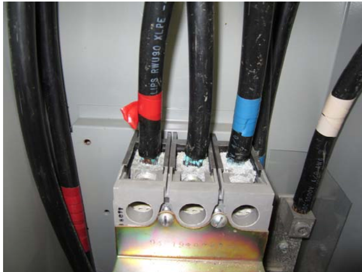
Photo 14: Well 6 - Severe corrosion on the line side wiring of the main disconnect box
