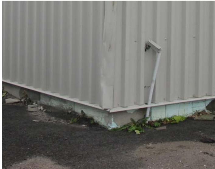
Photo 11: Well 5 - Damaged conduit
