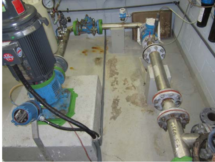
Photo 8: Well 5 - Corrosion of unprotected steel bolts
