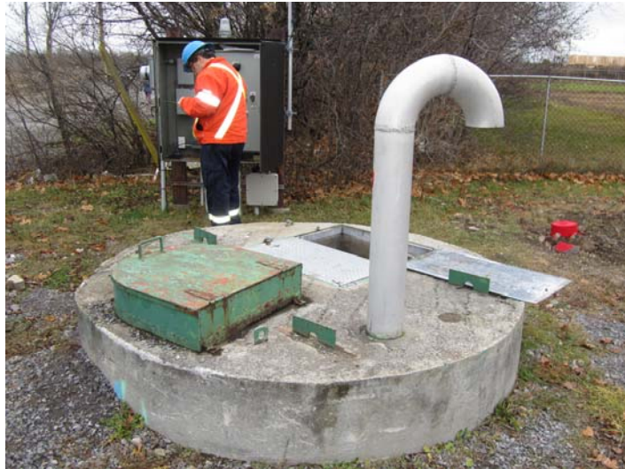
Photo 25: Robert Street SPS - Corroded access hatch cover
