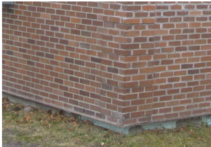
Photo 3: Well 3 - Cracked parging
